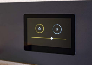
Touchscreen to regulate light and ventilation
